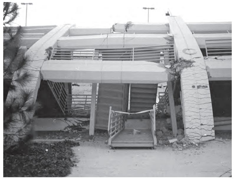
FILE PHOTO / DAILY SUNDIAL The 1994 Northridge Earthquake destroyed buildings throughout the San Fernando Valley, including structures on campus.
