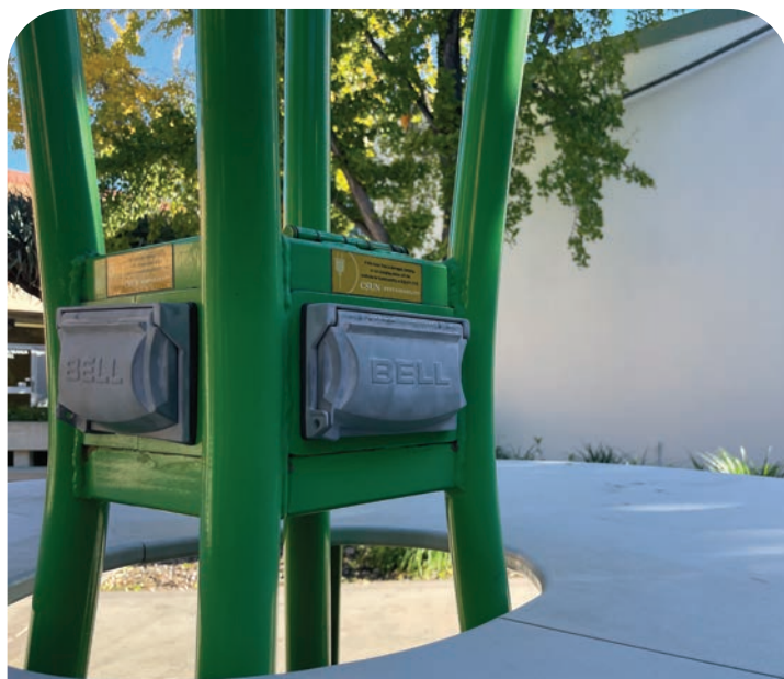
Solar powered phone charging station and rest area located in Jacaranda quad at CSUN campus in Los Angeles, Calif.
